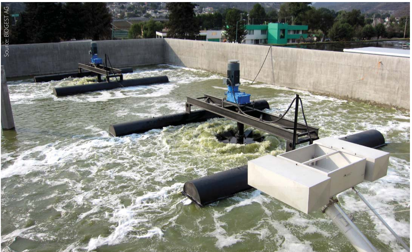
Figure 1: WWTP in Latin America: Aeration phase with surface aerators
